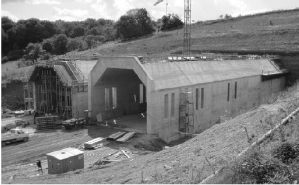
Figure 27 Construction of sonic boom alleviation section on the Finnetunnel tunnel in Germany (76)
