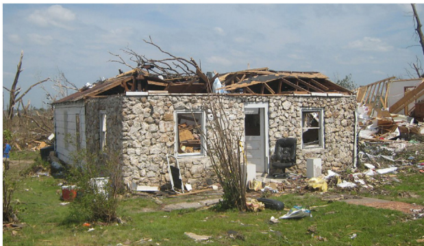
FIGURE 6 | Partial hip roof failure in Region 2 (image source: Dr. David Prevatt).
