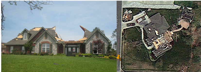
FIGURE 5 | Example of typical hip roof failure in Region 1, including an aerial photo showing the footprint of the partial failure (image source: Dr. David Prevatt, Google Earth).
