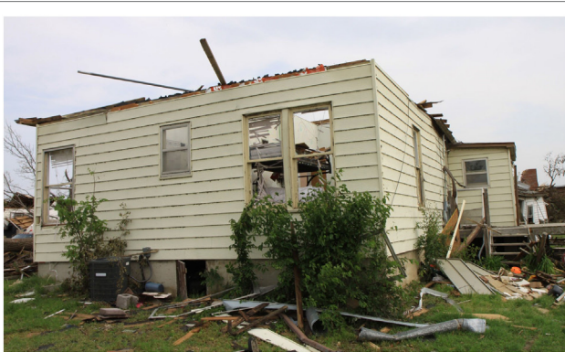
FIGURE 2 | Example of roof-to-wall-connection failure, corresponding to DOD-6 (image source: Dr. David Prevatt).
